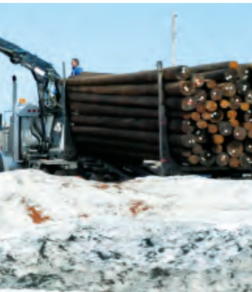
Top left: As the week progressed, working conditions improved as the ground continued to dry out. Bottom left: An empty lot in Center was utilized as a staging area for contractors to pick up poles.
